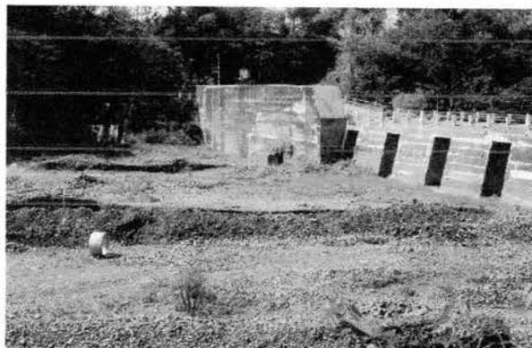
Figure 2. SABO Dam Condition After Eruption 2010 and Dredging
