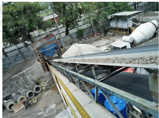
Conveyor Transfer Hopper ke Bin Material
