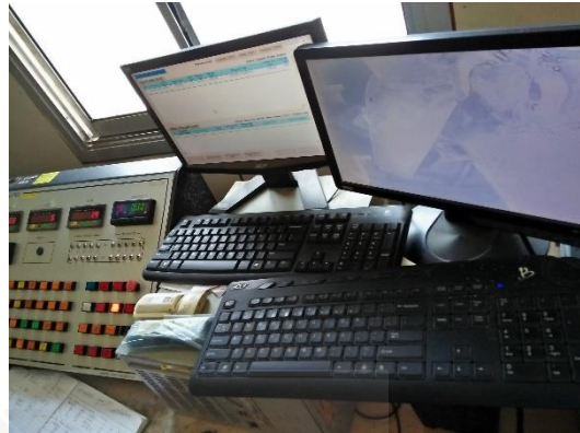
Control Panel Batcher
