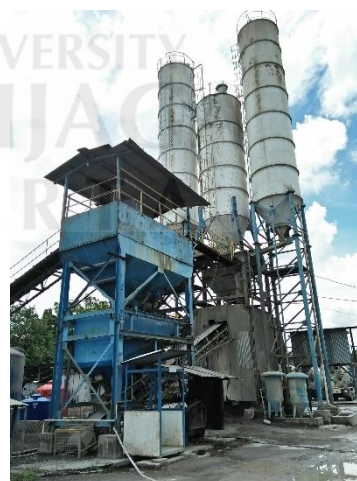
Mesin Batching Plant
