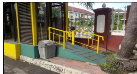
Figure 1. Ramp in Trans Jogja Shelter is Obstructed by Trees
