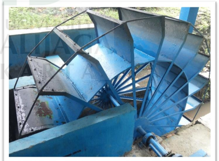
Gambar 2.19 Turbin PLTMH Singosaren, Bantul
