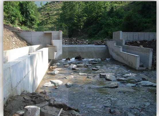
Gambar 2.7 Intake PLTMH Singosaren Sumber: https://adienergy.files.wordpress.com
